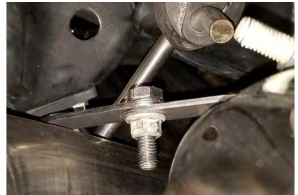
Detail 10b: Rear pipe hanger above front pipe hanger
